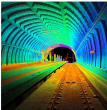
TrackSight™ LiDAR scan — real-time point cloud imaging inside a rail tunnel.
